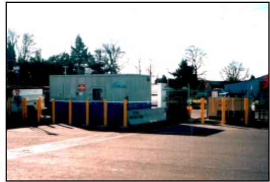
Compressor station housing at USF Reddaway.
