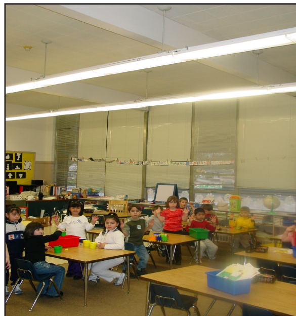
Stayton Elementary School improved its lighting with funds from Nike and SB 1149 funds.
