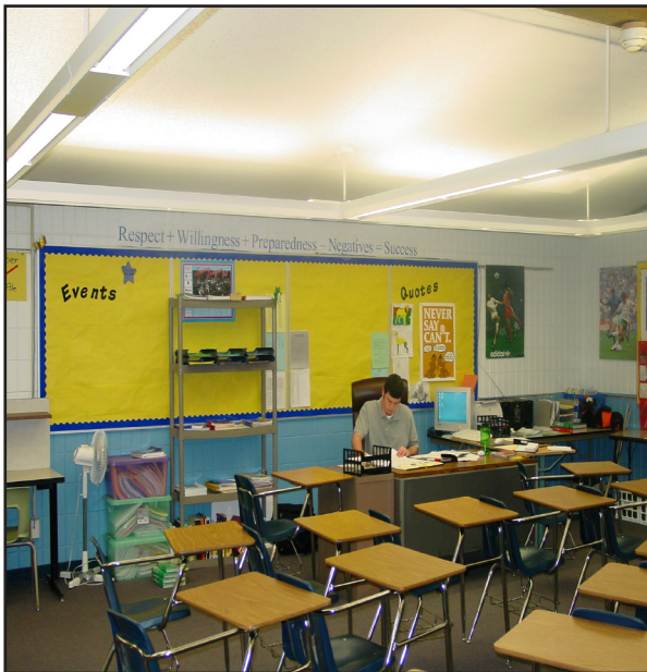
New lighting does not flicker or hum like the previous lighting. The light quality improved too
