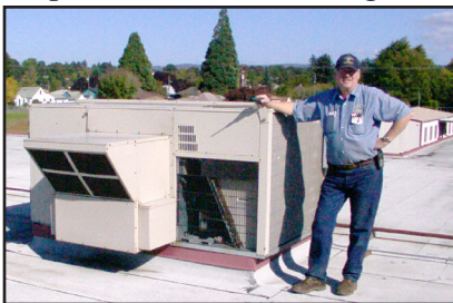
Ron Osborne, manager of the energy installation projects for North Santiam School District, shows off the roof top unit at Stayton Elementary School.
