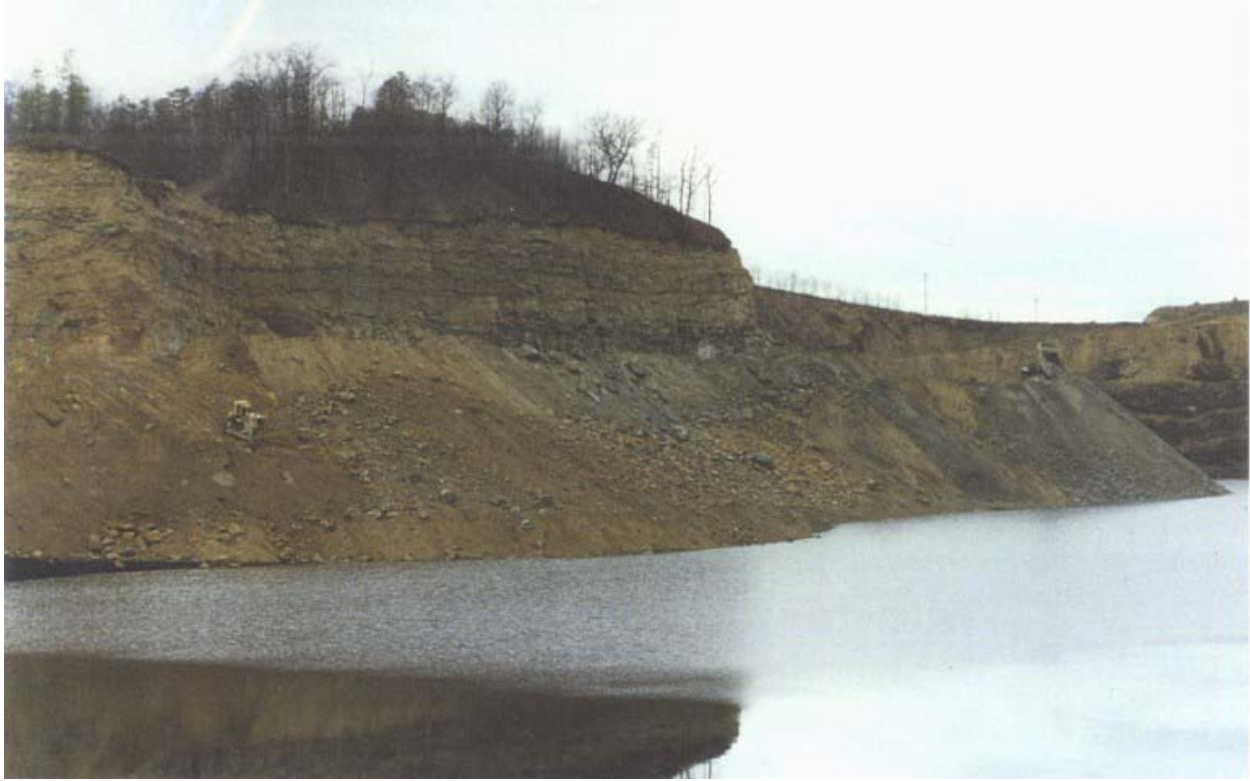
Photo 11. Construction of Seepage Barrier (Long View of Dozer and Truck) - March 6, 1995. Source: GAI. The work is being conducted at the southwest side of the impoundment. Pool elevation 1,000 feet msl. Mine roof elevation 964 feet msl.
