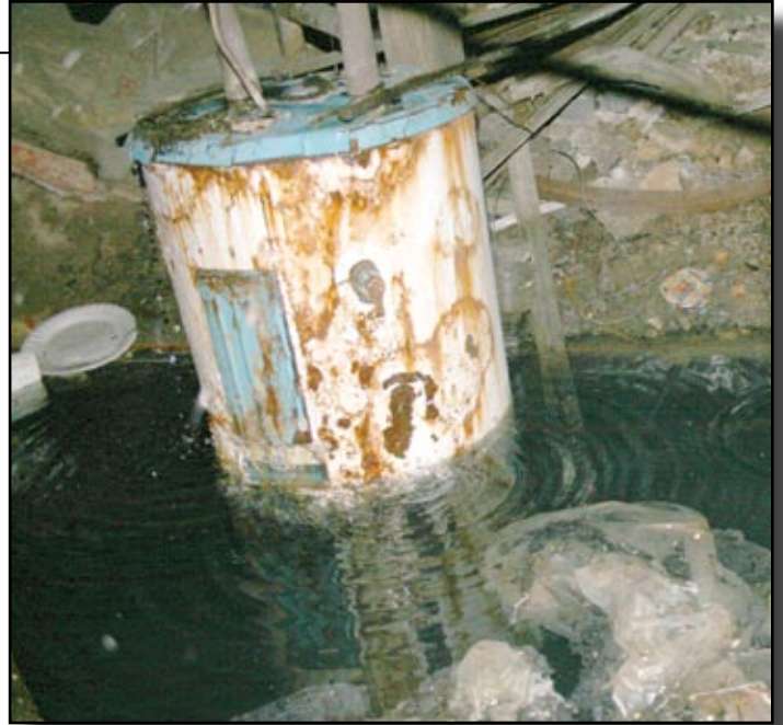
This hot water heater sits in 3 feet of water. You can see the water coming out of the top of the unit, which is compounded by leaking waste water pipes in the basement.
