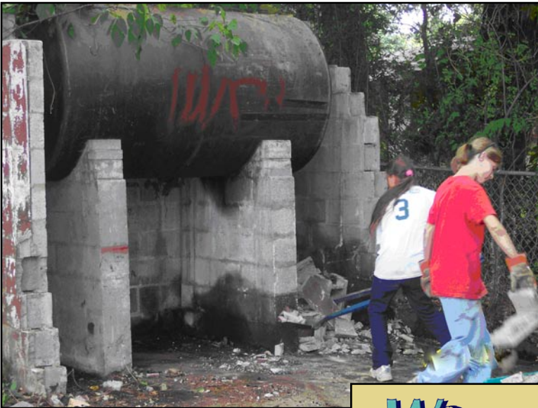
Volunteers demolish an unsafe structure at the back of a property on 4th Street
