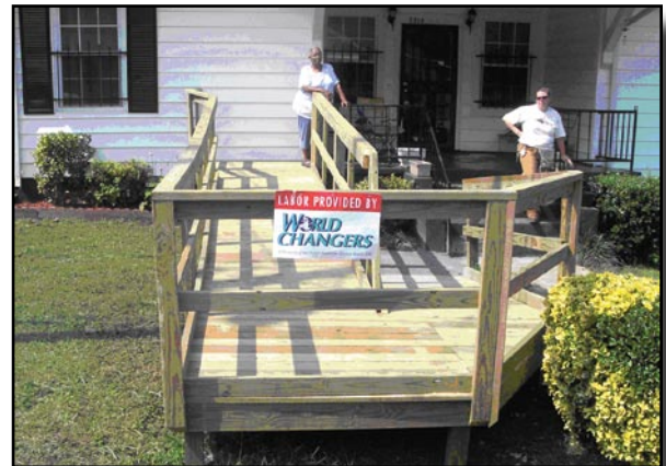
Handicap ramp built by World Changers last year on Gilbert Street in Chattanooga
