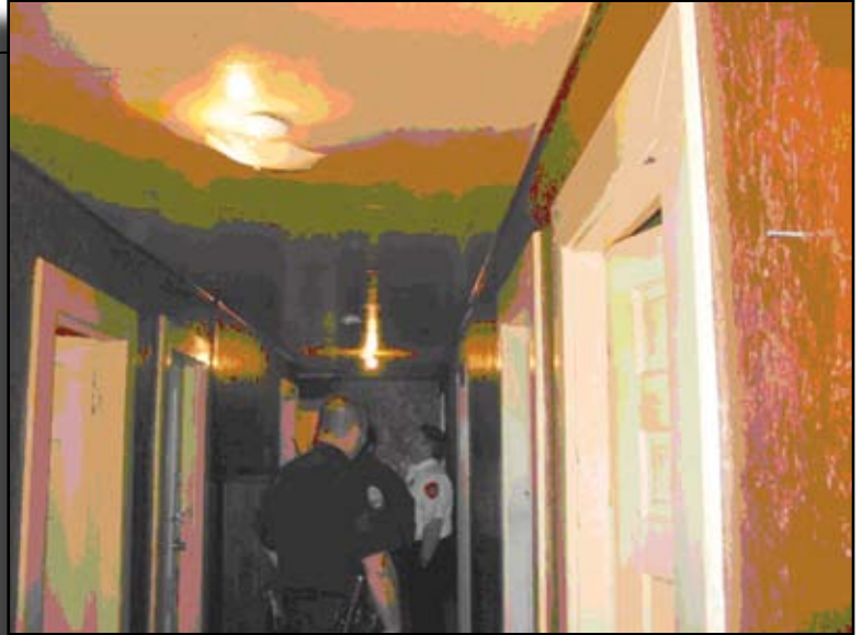
This single family dwelling was illegally converted to a boarding house. Plywood and doors were constructed to divide larger rooms into 10 small rooms large enough for little more than a mattress.
