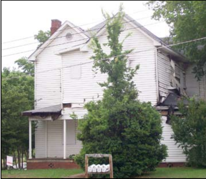
This property at 1401 Union Avenue has extensive fire damage, and the owner is in bankruptcy. It is slated for auction. Bankruptcies and foreclosures have similar maintenance issues.
