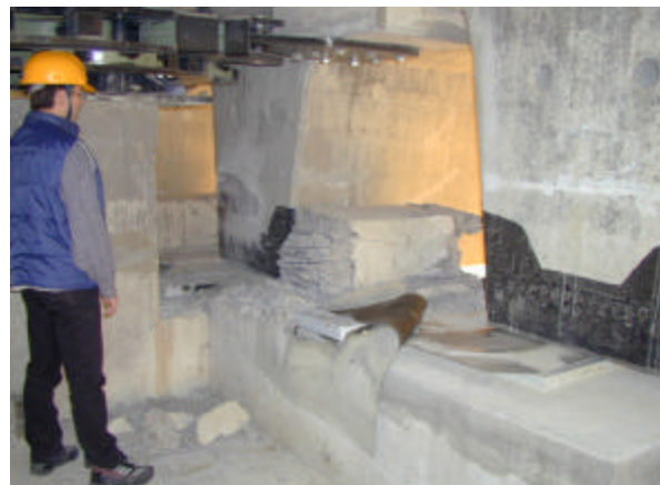
Figure 19. Shear block damage (translational restraint).
