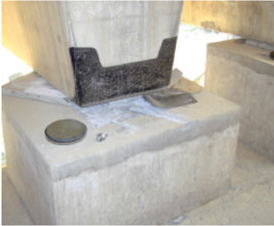
Figure 17. Typical dislodgment of bearing systems.
