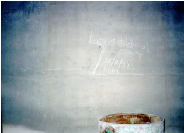
Figure 35. Longitudinal cracking of concrete liner
