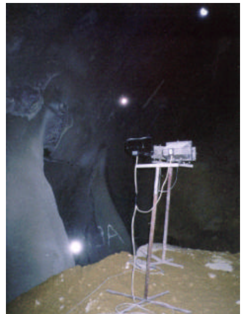
Figure 34. Spalled shotcrete at sets.
