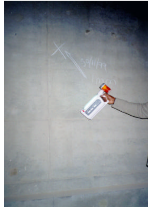
Figure 36. Radial cracking of concrete liner
