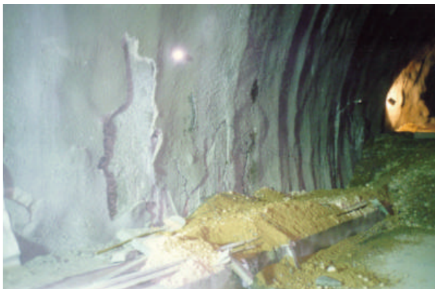
Figure 33. Spalled shotcrete liner segment.
