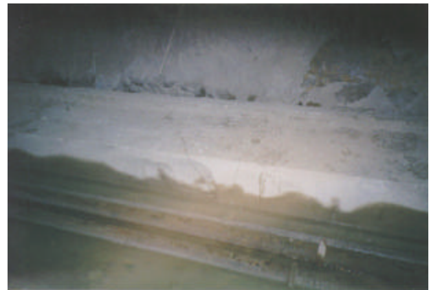
Figure 37. Utility box beam cracking.
