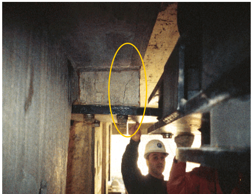
Figure 27. Incipient failure of EDU anchorage point.
