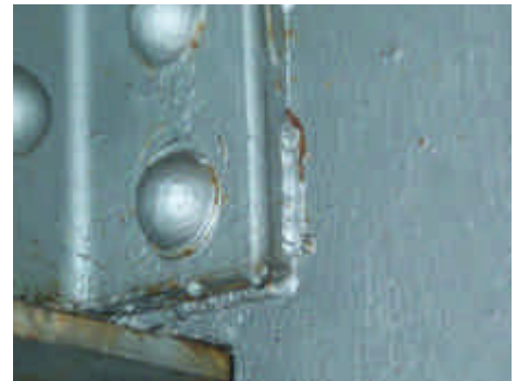
Crack indication in a tack weld.
