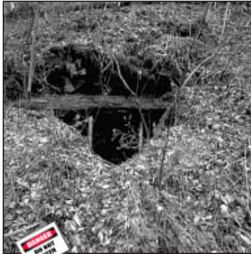
This is an abandoned underground coal mine entrance in Eastern Kentucky. It would be VERY dangerous to enter this mine opening. The unstable roof is caving in and large sections are continuously falling.
