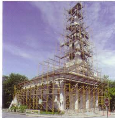
Collaboration between the Blackstone Valley Tourism Council, the National Park Service, and regional and state political leaders brought about the Blackstone Valley National Heritage Corridor, a place where a wealth of historic structures are receiving the care they need to stand as a reminder of the past for many more years.
