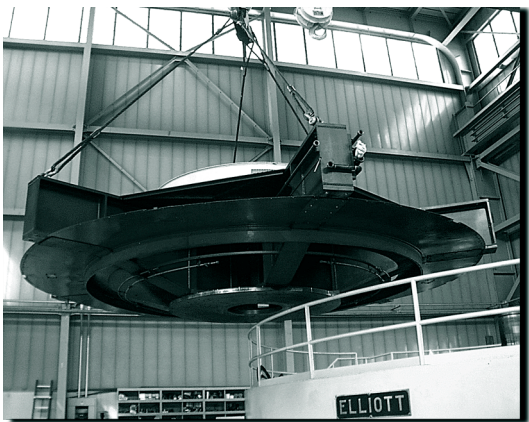
The Alcova Powerplant Generating Unit No. 2 undergoes replacement of a major component (photo by Reclamation).
