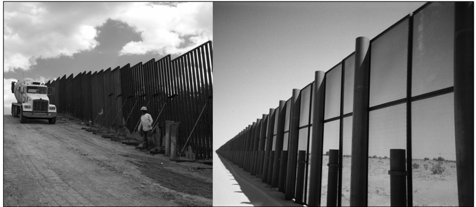
Figure 4: At Left, SBInet Fencing Being Deployed at Sasabe, Arizona; at Right, SBInet Fencing Deployed at Yuma, Arizona
