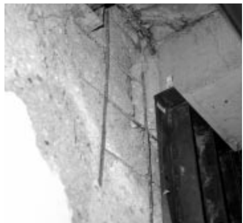
A deteriorated wall on the 15th floor, seen here with reinforcement bars and steel brackets, has been repaired.
