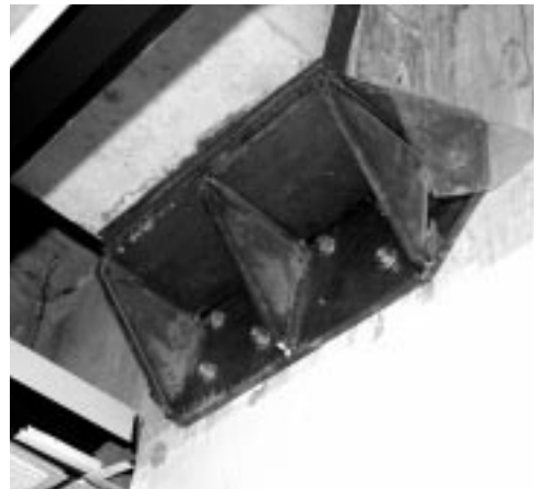
A typical steel bracket used to support crossover beams until permanent repairs are completed.
