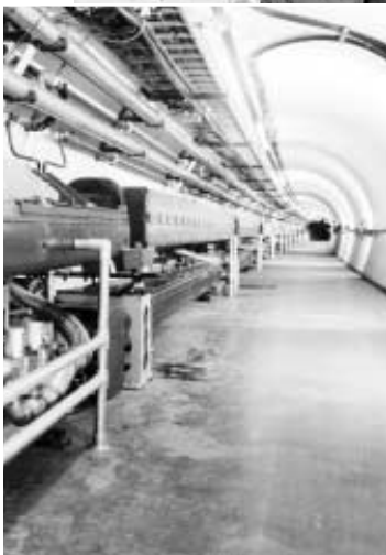
This is how the Main Ring/Tevatron tunnel looked before crews began dismantling the Main Ring accelerator.
