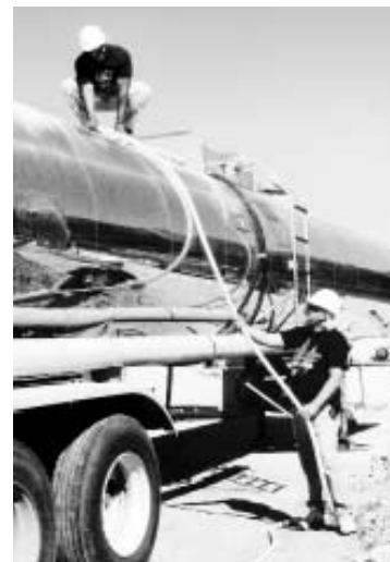
Bob Slazyk (right) and Drue Wallace, of the Mechanical Support Department, drain low-conductivity water from the tunnel into a 7,000-gallon tanker.
