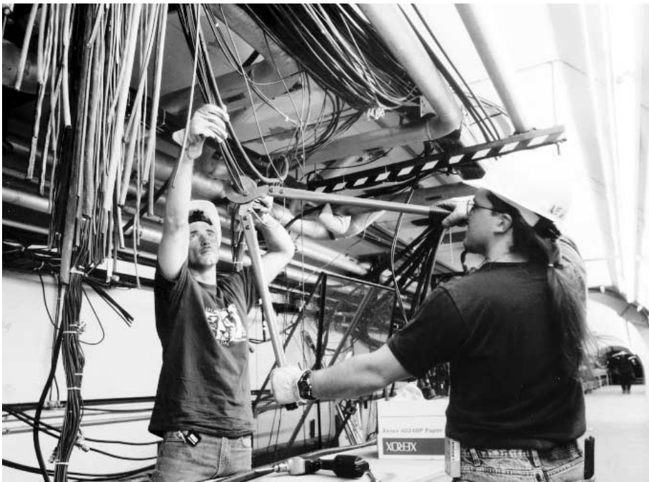
Chuck Broy (left) and Dwayne Newhart, both operators who have been recruited for demolition work, cut out cables from FZero.
