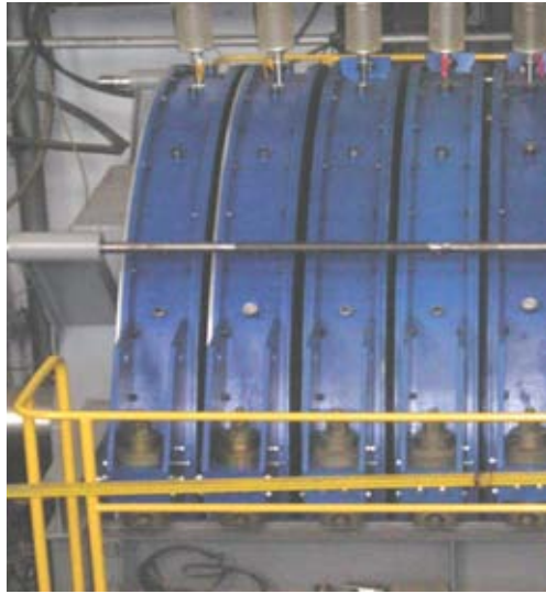
Figure 3.21. Photograph of five LTD cavities assembled in a voltage adder configuration out of the planned ten 1-MA, 100-kV LTD cavities that will complete a 1-MA, 1-MV voltage adder.
