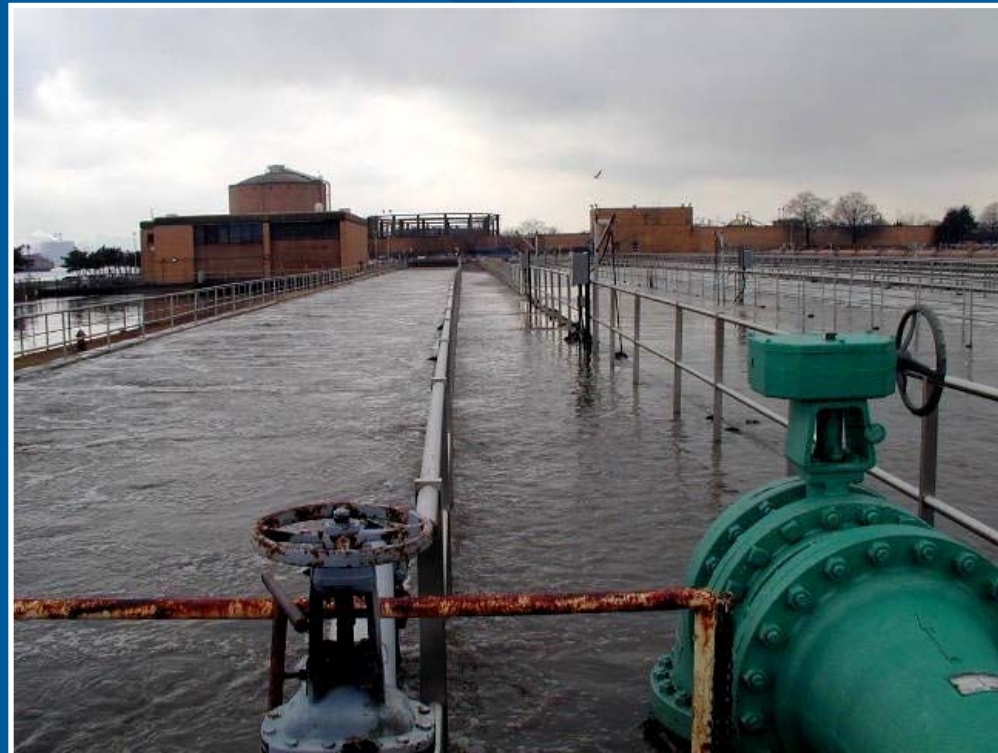
Treated Sewage Backed-Up at a Bronx WPCP
