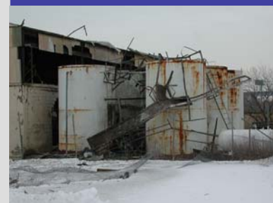
Figure 1. Damage to the north side of the ASCO facility.*
