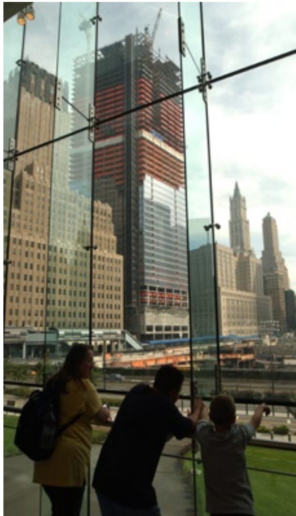
Construction continues at Seven World Trade Center, which was destroyed during the attacks on September 11, 2001.
