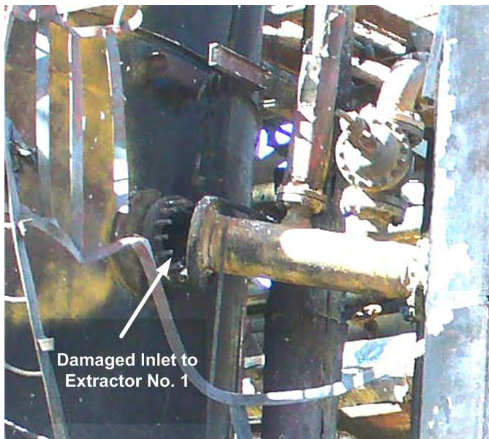
Figure 8. Damaged 10" propane inlet on Extractor No. 1
