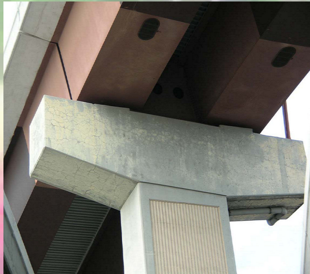
Cracking due to ASR in a five-year-old bent cap with high cement factor and no preventive measures. Sent by: Brian Merrill, Texas DOT
