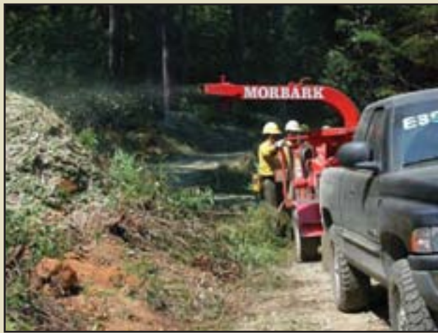
Figure 5.72 – Slash material can be chipped on site to reduce fire hazards and increase line of sight. In this photograph, brush and trees on cut slopes are cut, chipped, and blown back on the slopes as mulch.
