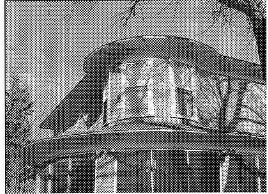
At 1123 Tijeras Avenue NW, details to be preserved include the turret, diamond-pattern window muntins, projecting roof with exposed rafter ends, and siding of wood shingle and clapboard.
