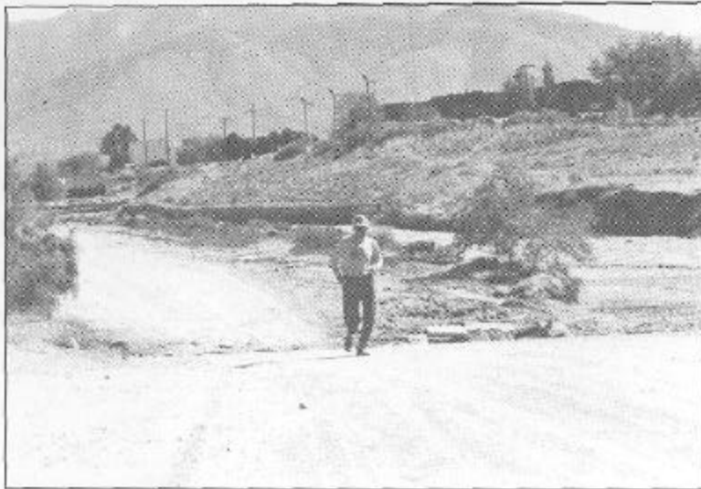
Road adjacent to arroyo in Arroyo Del Oso Park
