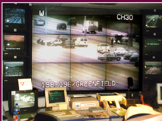
MICHIGAN INTELLIGENT TRANSPORTATION SYSTEMS CONTROL CENTER
