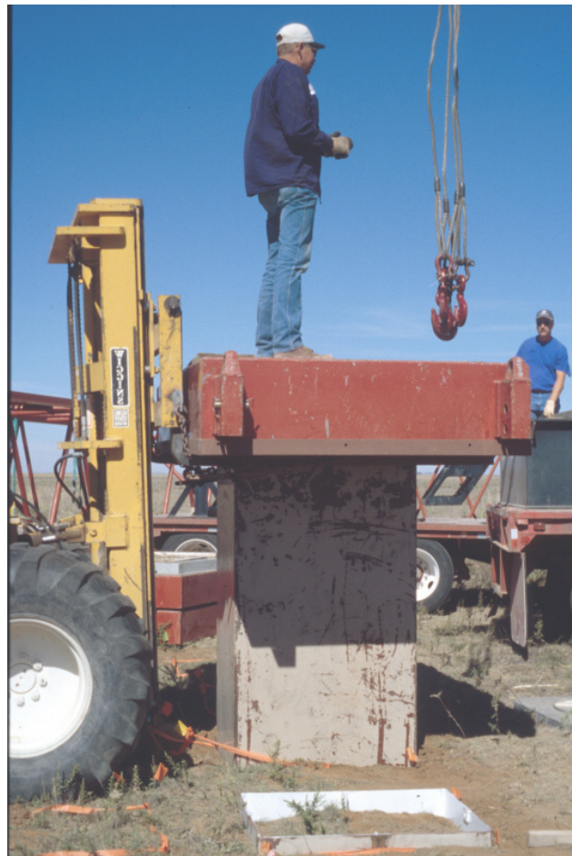
Figure 4. First weight on top of lysimeter box while forklift maintains alignment and controls rate of downward movement.
