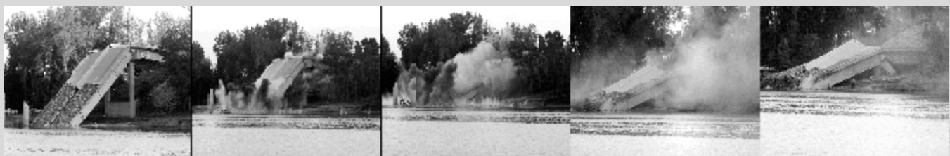
Demolition of the fallen bridge structure began on June 2. The task was somewhat delicate, as existing structure was very close by.
