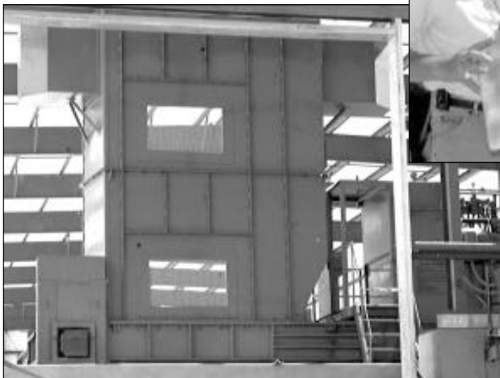
The backside of TRU Blue has two windows so Lab employees can see the inner workings of the machine as it cuts and crushes the metal waste. Insert: John Loughead of Solid Waste Operations (FWO-SWO) holds a mock-up of what the metal waste will look like in the end: a home plate-shaped puck weighing about 80 pounds. Photos by LeRoy N. Sanchez
