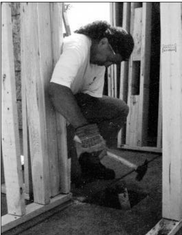
Jerry Romero of Physical Chemistry and Applied Spectroscopy (C-6) works to secure a wall to the foundation of a Habitat for Humanity site in Española. Romero is one of many Lab employees who volunteered weekends in an effort to complete the first in a series of low-cost houses constructed by the Española Valley/Los Alamos Chapter of Habitat for Humanity. Photo by Michael Carlson
