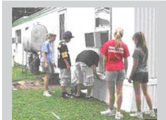
NRCS Earth Team volunteers perform hands-on home-repair projects for needy families during the Delaware Bay Workcamp
