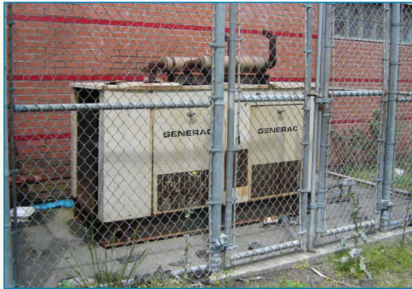
Figure 4-47: Generator mounted at grade level damaged by flooding
