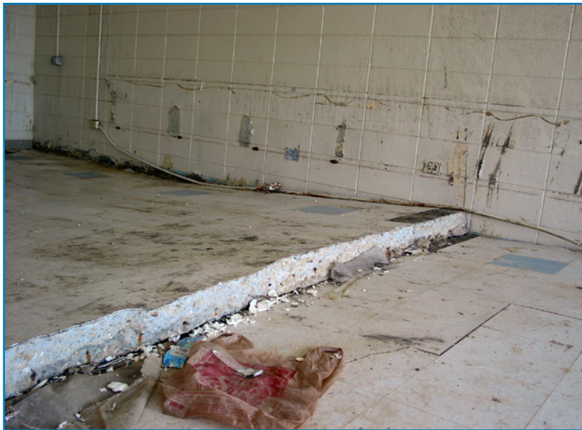
Figure 4-23: Cracked concrete floor slab at Charles B. Murphy Elementary School
