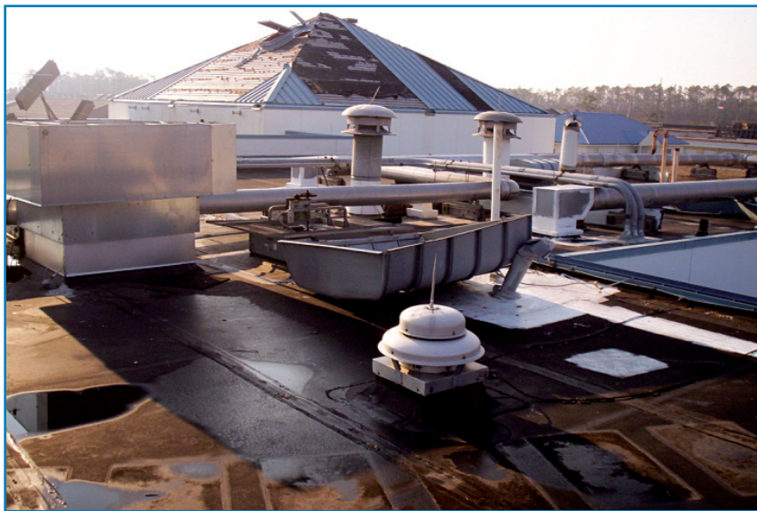
Figure 4-8: Roof damage on Hancock Medical Center
