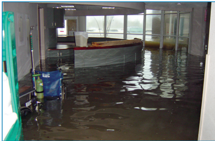
Figure 4-3: The lobby of Hancock Medical Center was under 3 feet of water.
