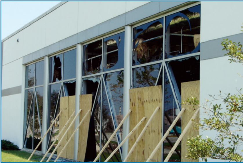
Figure 4-10: Broken windows at West Jefferson Medical Center
