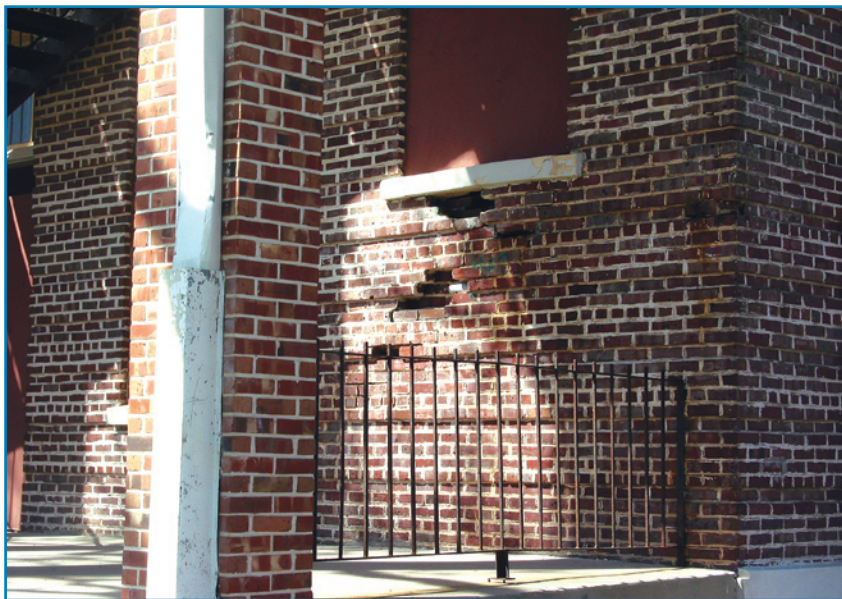
Figure 4-26: Cracked brick veneer at St. Stanislaus High School
