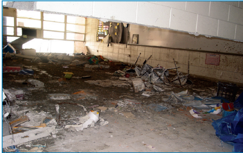
Figure 4-30: Interior damage at Charles B. Murphy Elementary School
