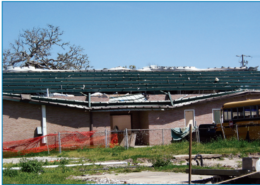
Figure 4-27: Metal roof covering peeled away at a St. Stanislaus campus building
