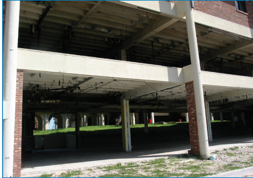
Figure 4-20: Lower floors washed away by the storm surge at St. Stanislaus campus
