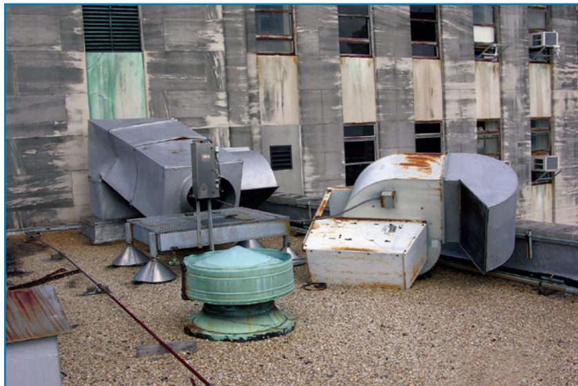
Figure 4-12: Topped HVAC equipment at Charity Hospital, New Orleans
