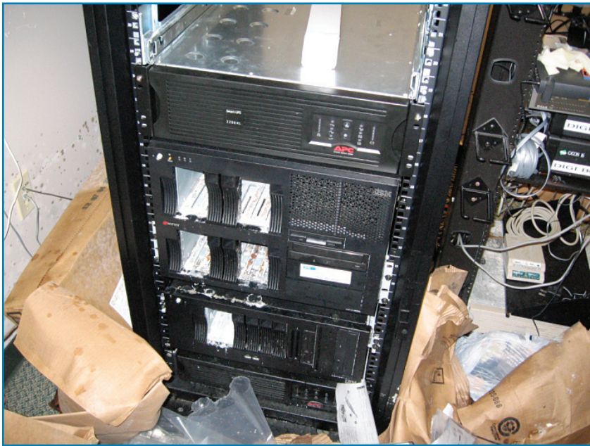
Figure 4-14: Damaged computer network equipment at Hancock Medical Center
