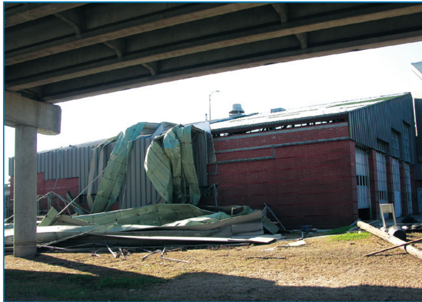
Figure 4-42: Metal roof and wall panels peeled off the Third District Fire Station in New Orleans
