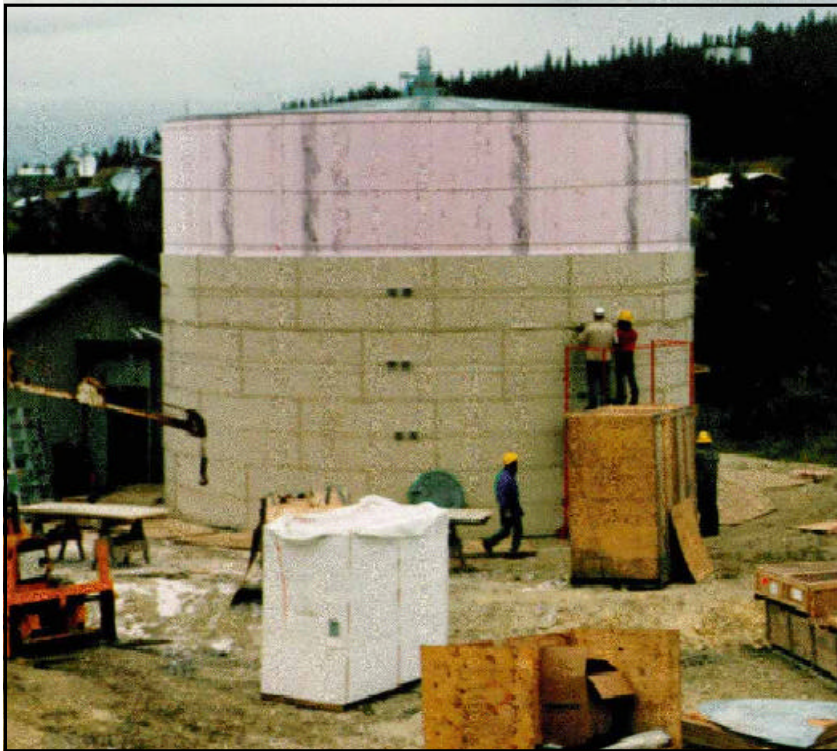
A storage tank under construction in White Mountain, Alaska, is encased in insulation to prevent water in the system from freezing. Constructing water systems to withstand extreme weather conditions is one reason Alaska Native Village systems have high per-household needs.
