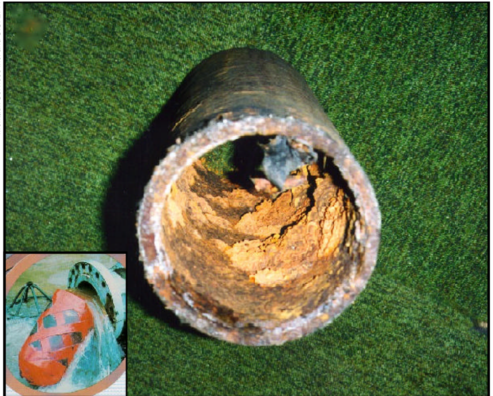
This pipe shows clear signs of tuberculation, a condition resulting from the accumulation of mineral deposits and debris. Tuberculation can reduce pipe capacity and impair drinking water quality. One method of removing tubercles involves sending a “pig” (insert) through the system to scour the sides of the pipe.
