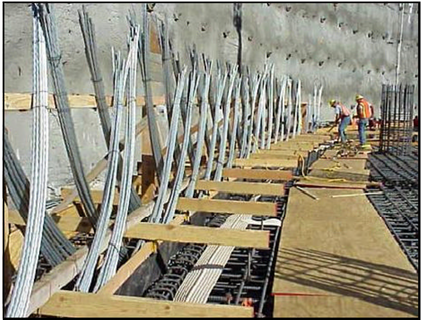
At a storage facility near Los Angeles, workers install seismic cables to provide structural resiliency for earthquake protection
