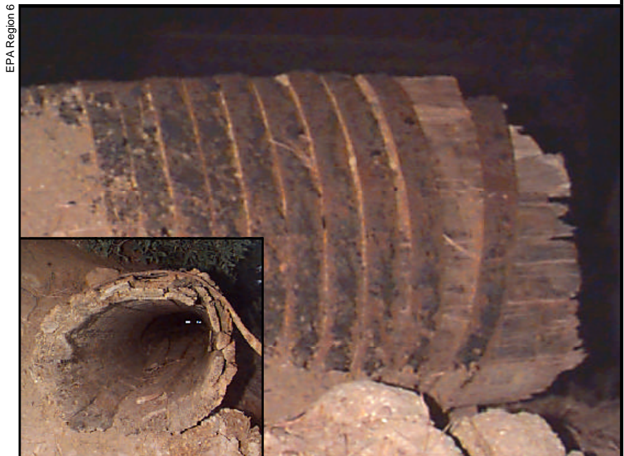
A section of wooden pipe dating from the early 1900s is removed for replacement by iron or PVC pipe. The service life of a water line can range from 10 to 200 years depending on the pipe material, soil type, and climate conditions.
