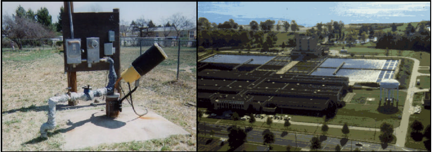
Water systems differ greatly in size and complexity, from a simple well pump with chlorinator (left) to a large-scale filtration plant.
