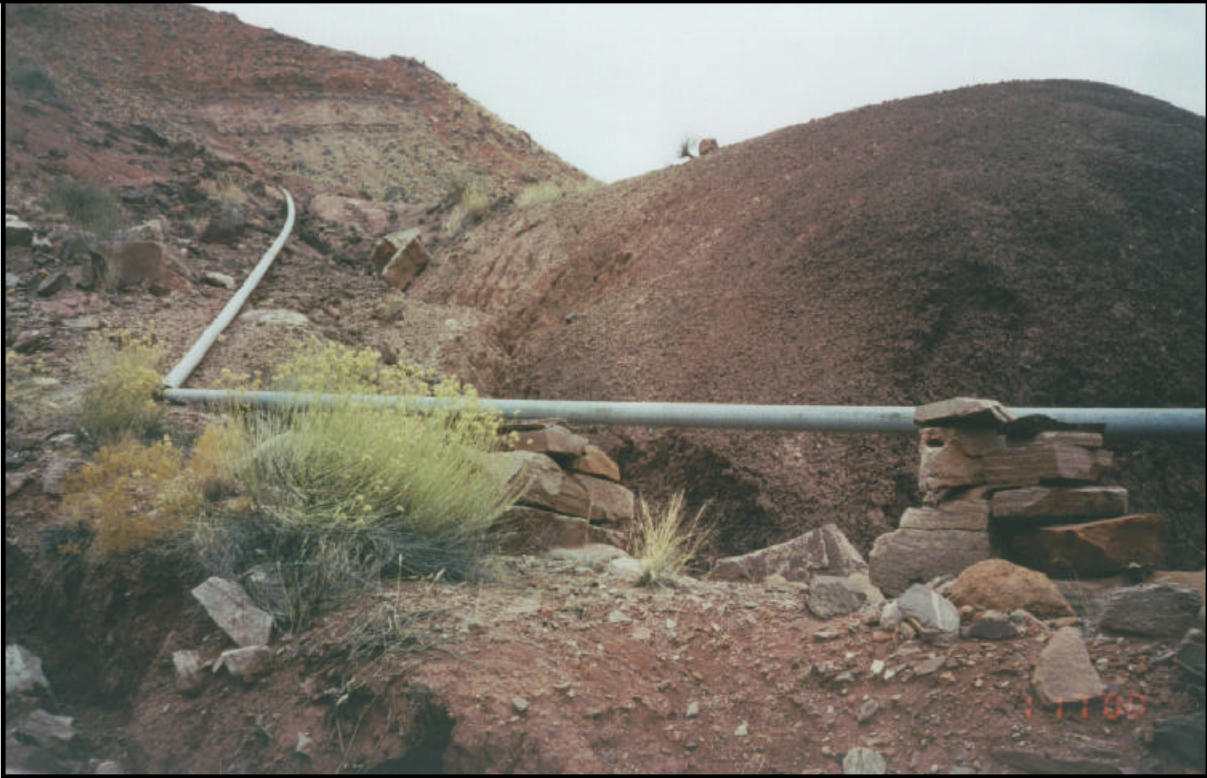
The expense of burying pipe leads some systems to develop expedient but precarious solutions such as the one pictured here. Water service will be disrupted if pipes are not buried or otherwise adequately protected.
