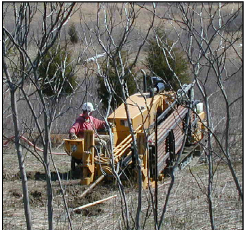
Pipe is installed to provide safe drinking water to homes in Rensselaer County, New York, that had previously used untreated water from a transmission line. The DWSRF contributed $4.9 million in funding assistance to this project.
