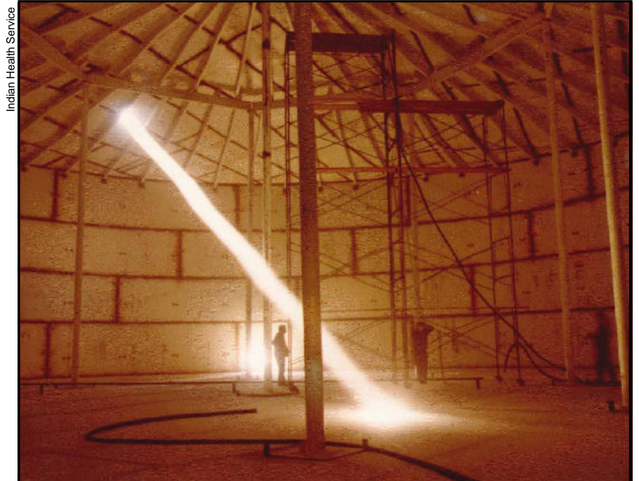
The construction of a treated water storage tank nears completion in Nuiqsut, one of the most northerly communities in Alaska. In many Alaska Native communities, water tanks and treatment plants must be elevated on pilings to prevent the heated facilities from subsiding into the permafrost.
