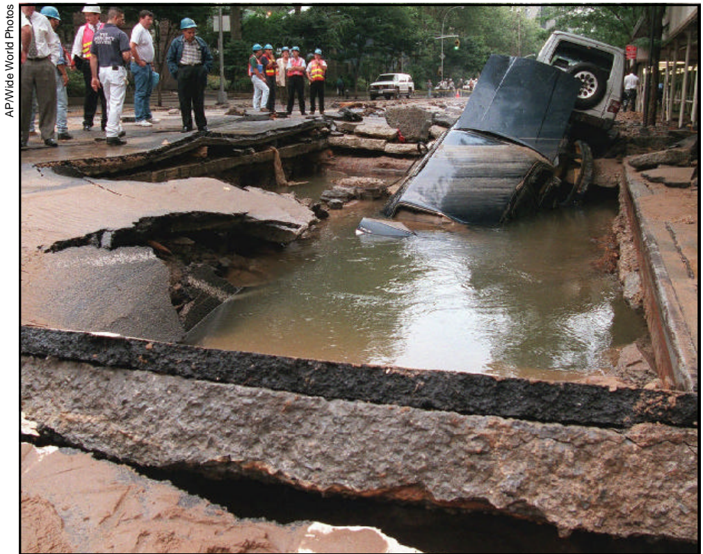
A ruptured water main in New York City closed a section of a major thoroughfare and limited service to two hospitals. The majority of the nation's distribution lines were installed in the mid-1900s. Towns and cities are finding it increasingly necessary to replace old and deteriorated pipe.
