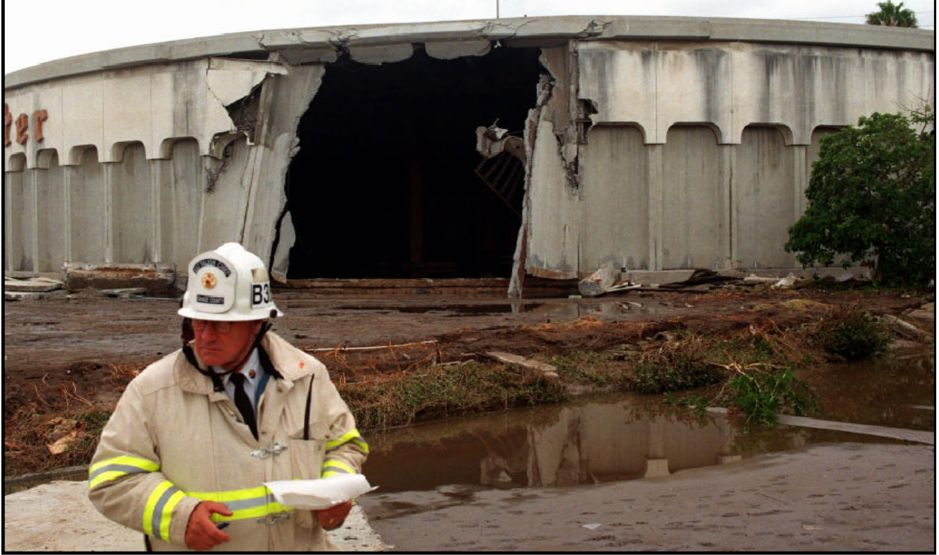
This 31-year-old storage tank ruptured in Westminster, California, sending a 6-foot wave of water through the city that damaged or destroyed about 50 buildings and over a dozen vehicles. Storage tanks should be replaced or periodically rehabilitated to preserve their structural integrity.
