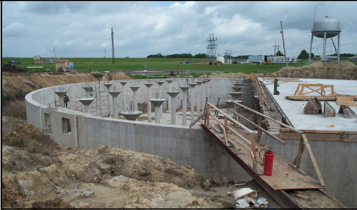
Corsicana, Texas, is increasing the capacity of its water treatment plant with a $10.8 million loan from the Texas DWSRF program. The expansion will allow Corsicana to extend service to the City of Frost where the State declared the water non-potable due to violations of health-based standards. Shown is one part of the plant expansion—the construction of a large clearwell that will provide the disinfection time necessary to inactivate harmful microbiological contaminants.
