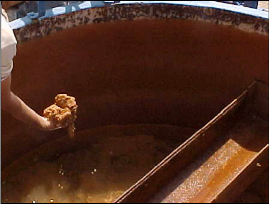
Filtration plants consist of a series of treatment stages, each of which is critical to the production of safe water. Shown is a filter bed that is clogged with mud and treatment chemicals. The clarifier that should have removed these particulates in the preceding stage is in poor condition and needs to be replaced.
