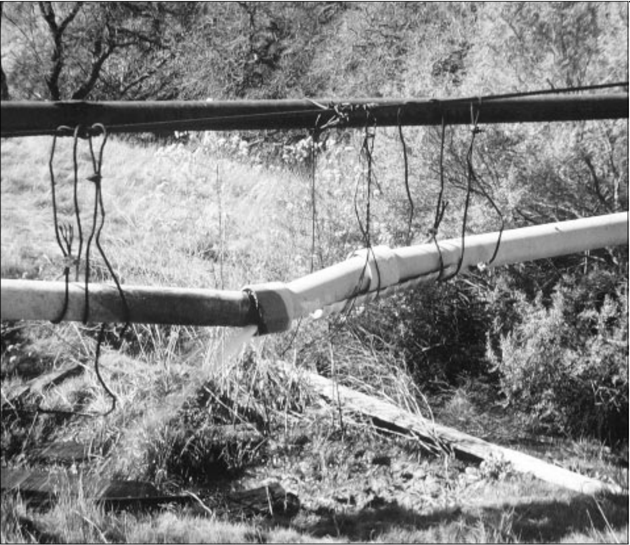
Emergency repairs to this transmission main make it possible to continue providing water. However, replacement is needed soon to avoid failure and the possibility of a water outage.
