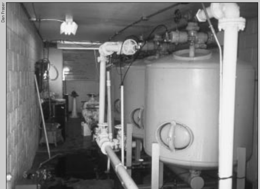
Pressure filters at Ethete
