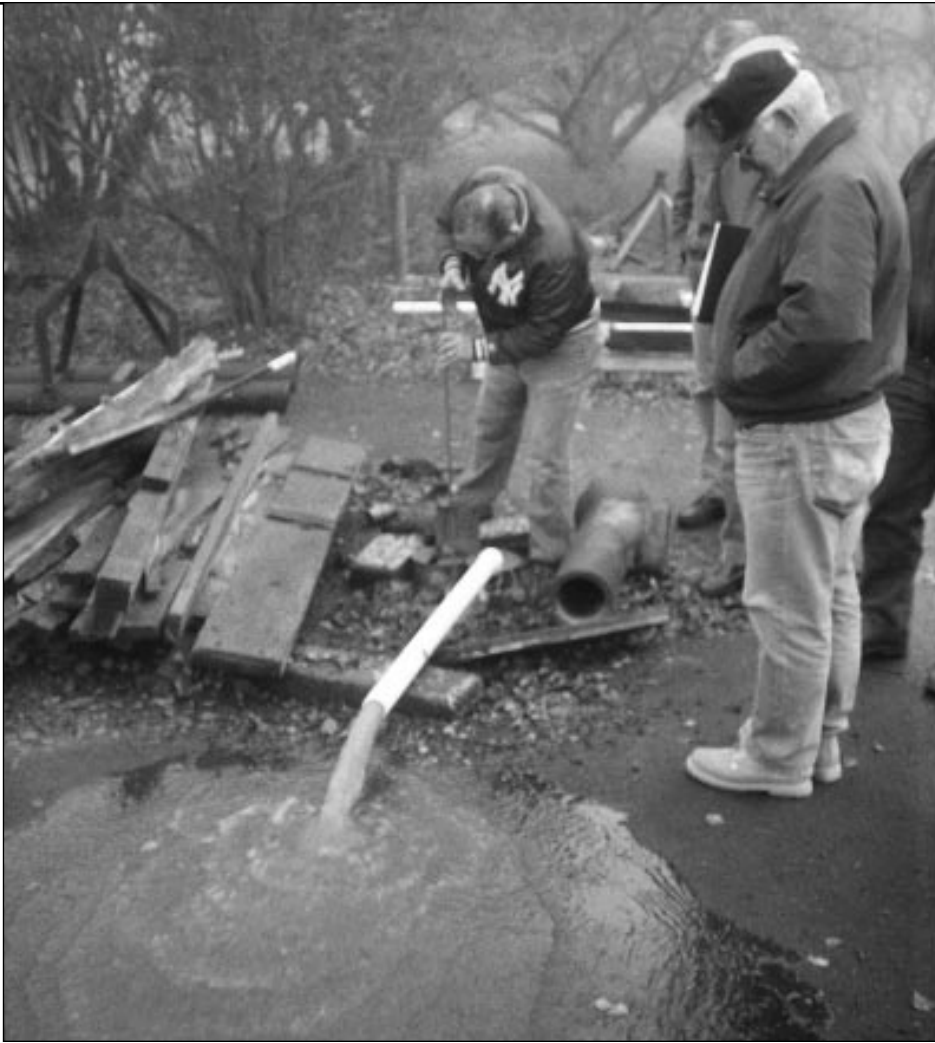
The small system operator shown above is flushing iron from the water system's distribution system. More than 3,100 small systems have an unmet need to treat for iron and manganese. These secondary contaminants make water reddish-brown and stain sinks and laundry.
