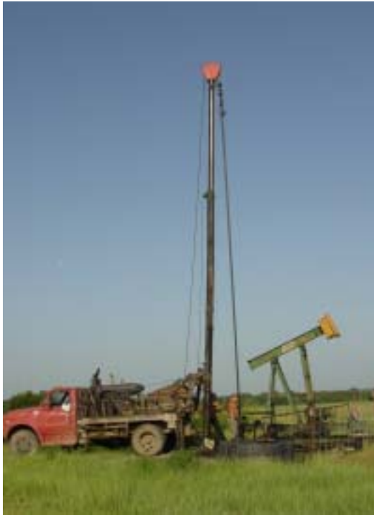
Running low-volume submersible pump, Beard Lease, OK.
