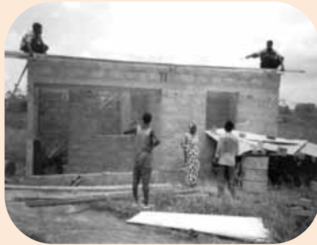
In Côte d'Ivoire, Maurice Djan Kouadio launched a Habitat for Humanity program as an outgrowth of his 1998-99 experience as a Humphrey Fellow at the University of Minnesota. The Habitat home under construction here was one of the 69 that volunteers built in Côte d'Ivoire.
