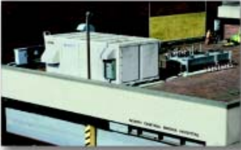
A 200-kilowatt phosphoric-acid fuel cell sits on the roof of the North Central Bronx Hospital.
