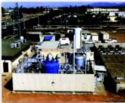
A Fuel Cell Power Plant
