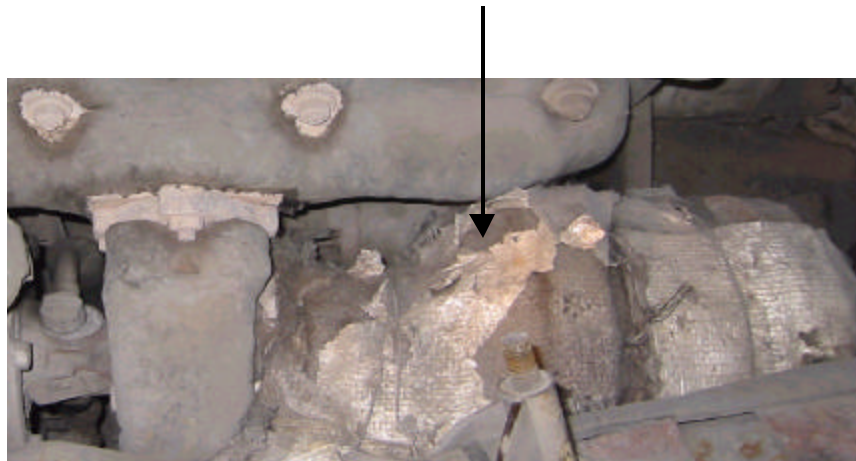
FIGURE 1. Worn Insulating Material Requiring Replacement
