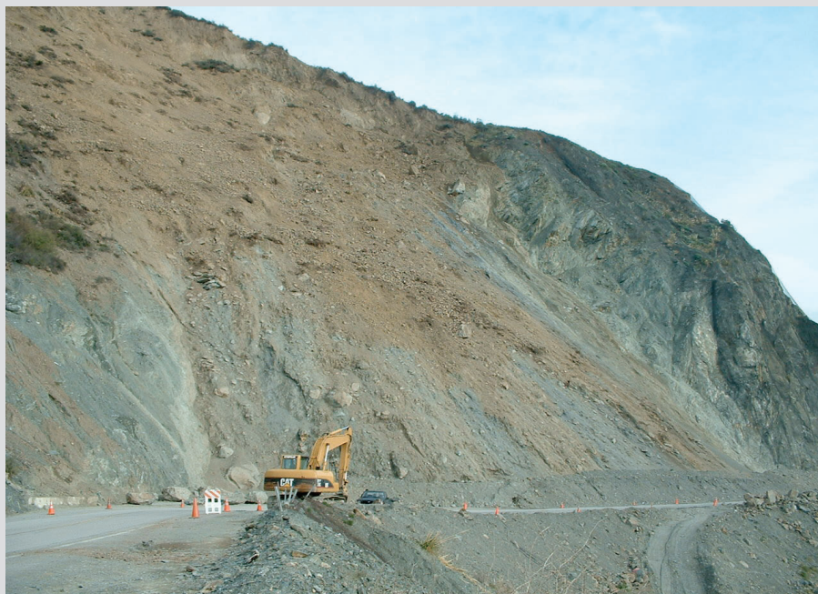
California Department of Transportation (Caltrans) crews work to reopen Highway 1 at Pitkins Curve during winter 2004. When this photograph was taken, one lane of the highway was still closed (note boulders at lower left behind the traffic barricade). This site is currently the most active landslide on the Big Sur coast. (USGS photograph by Cheryl J. Hapke.)
