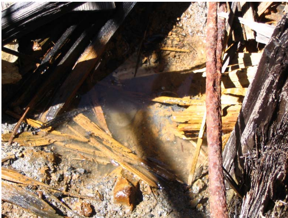
4. Free elemental mercury under debris and water at the mill works building.
