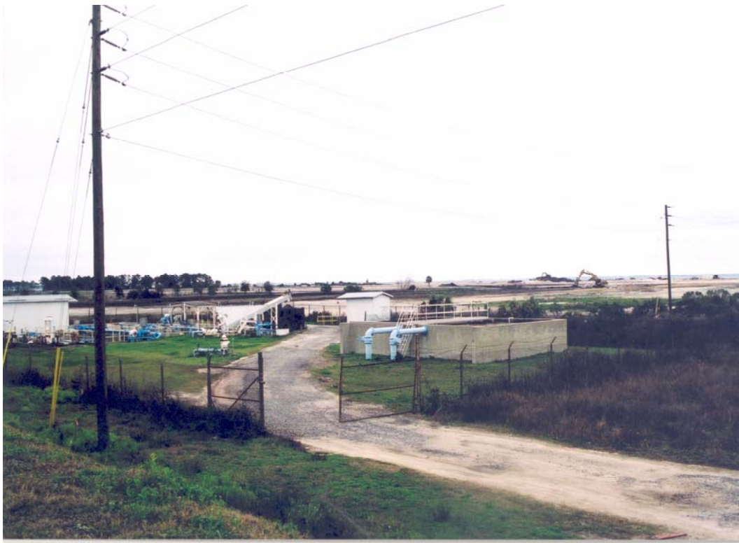
Photo 8: View to the southwest from the bridge, remediation equipment on the southern parcel in the distance.
