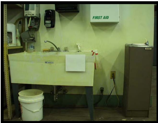
Figure 4. Yellow staining was observed on the plastic sink, outlet cover, and wall surfaces.
