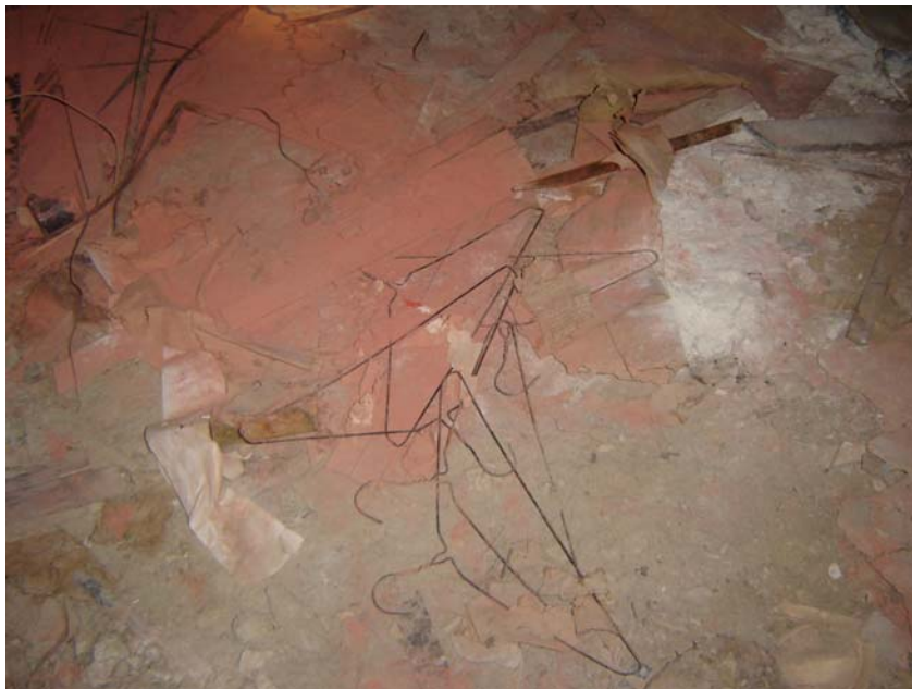
Close-up of crawl-space floor. Note the residual white, powdery DDT and hazardous substance debris covering the floor space.
