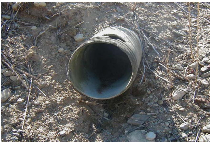
Open Pipe (Safety Hazard) in Former Lagoon Area.
