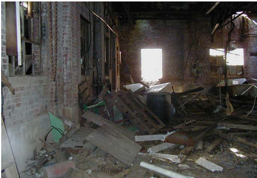
Interior of Main Process Building
