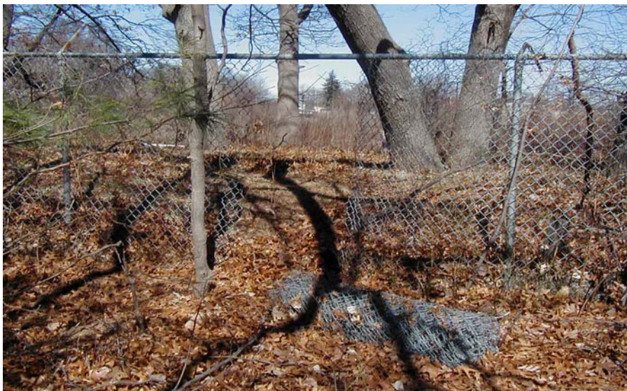
Breach in fence along northern property boundary.
