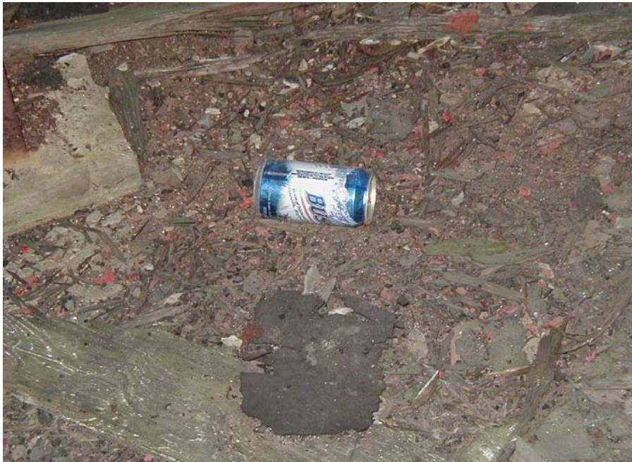
Interior of Main Process Building – Evidence of Trespassing
