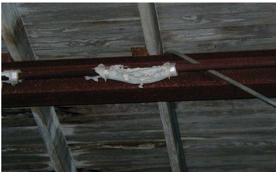
Interior of Main Process Building – Pipe Insulation
