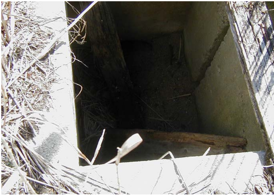
Open Catch Basin (Safety Hazard) in Former Lagoon Area.
