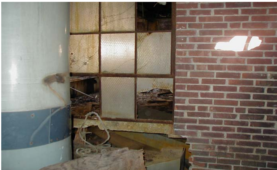
Exterior of Main Process Building – Broken Windows
