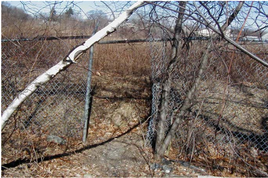
Breach in the Fence along Northern Property Boundary
