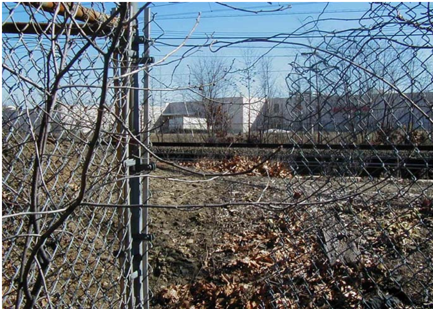
Breach in the Fence along Northeastern Property Boundary (Former Raymark Site is visible across railroad tracks).
